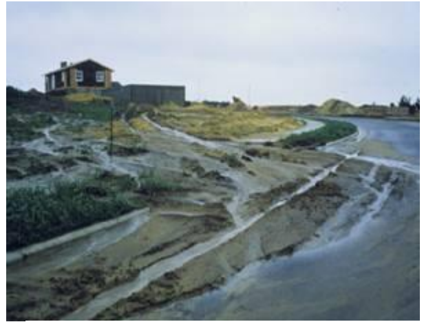
Improper Stormwater Runoff Control
