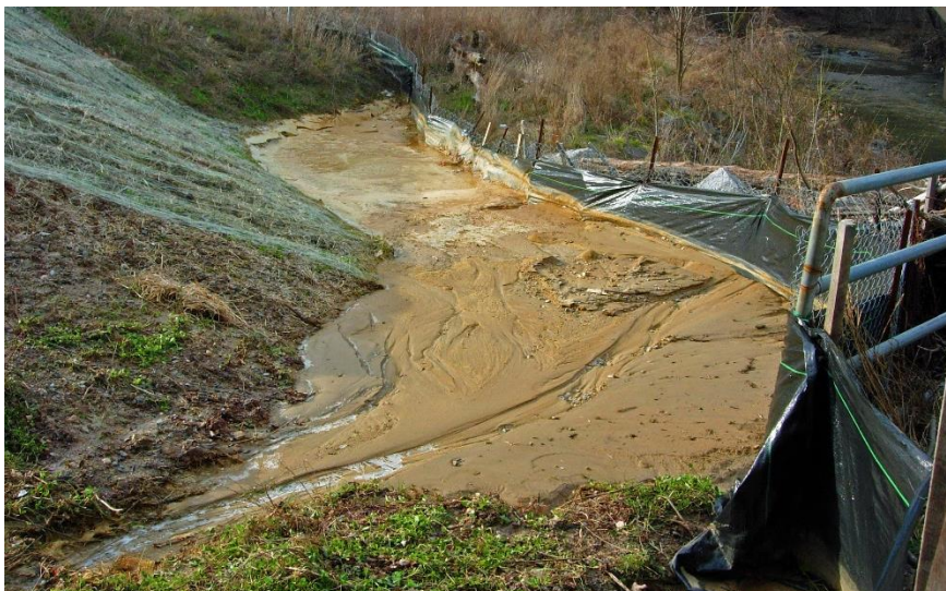
Soil erosion and sediment runoff during construction
