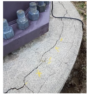
Failing concrete in a caisson foundation.
