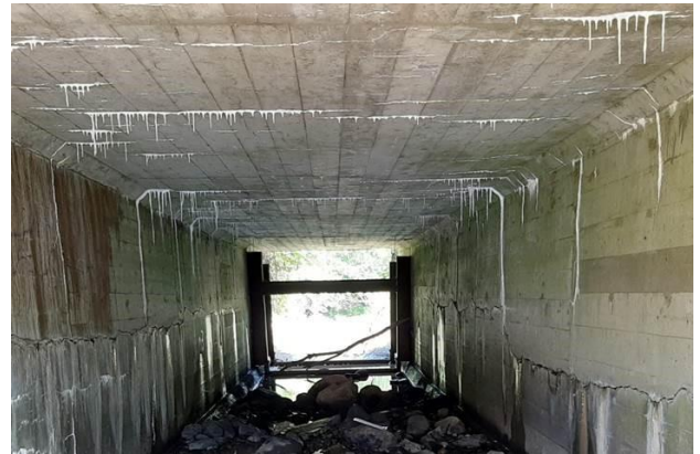
Box culvert with cracking and efflorescence caused by ASR.
