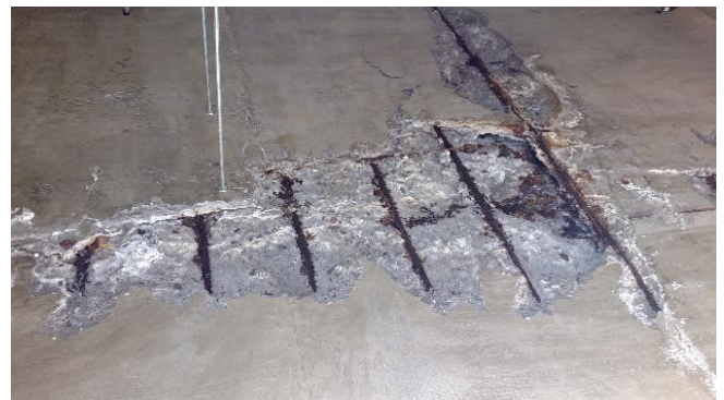
Slab delamination due to reinforcement corrosion.
