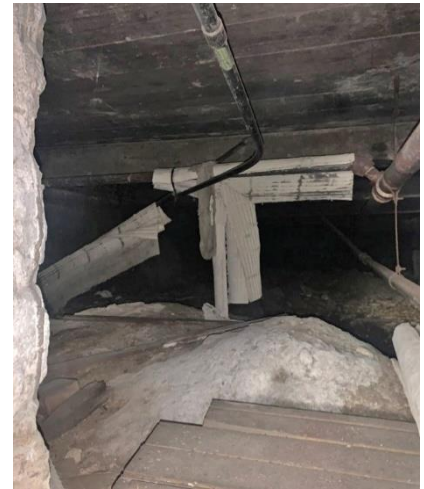
Disturbance of Pipe Thermal System Insulation (TSI) within a crawlspace.
