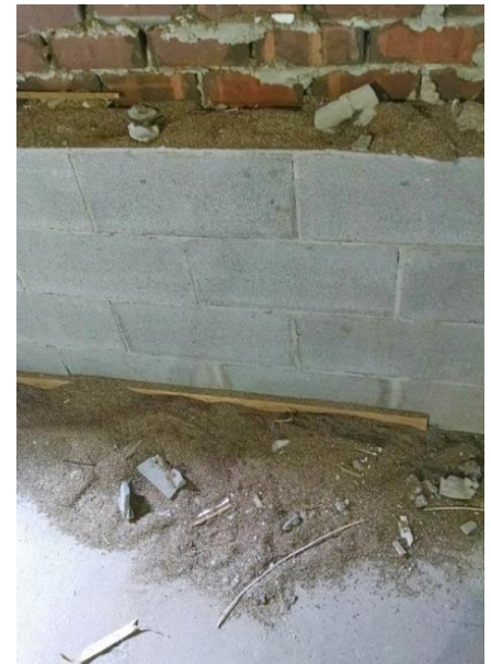
Loose Fill Vermiculite from a Concrete Masonry Unit (CMU) Wall.
