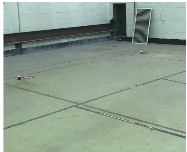
Mercury containing gymnasium floor prepped for wipe samples.
