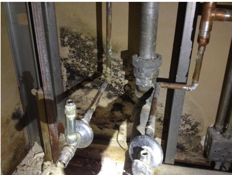
Mold discovered within a wall cavity during renovation work.
