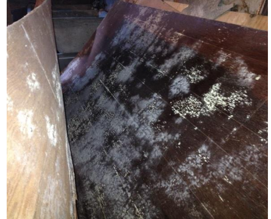
Fluorescent mold on stored materials within a basement area.
