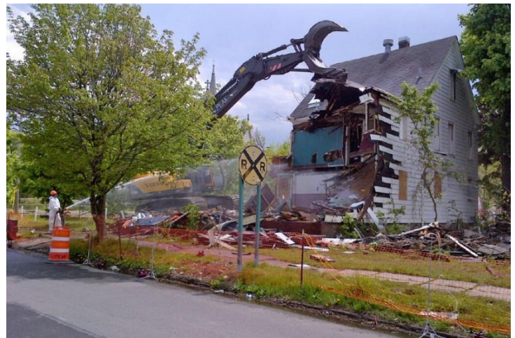
Example of a demolition with asbestos in-place for a vacant residential building.
