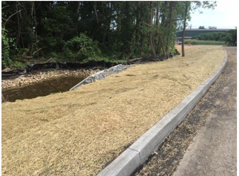
Proper Construction Phase: Rolled straw seed blanket installed following final grading of topsoil.
