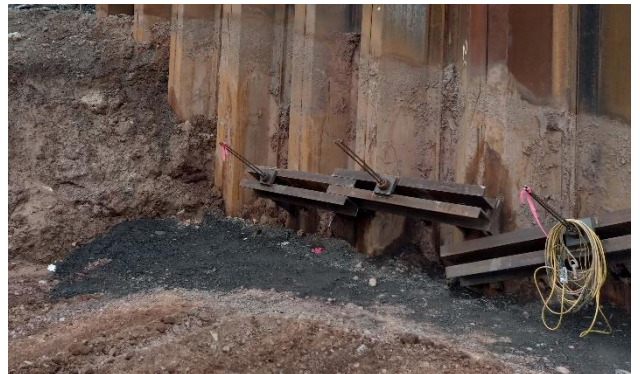
Corrosion of Buried Steel Structure
