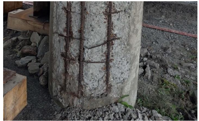
Corrosion of Buried Concrete Structure
