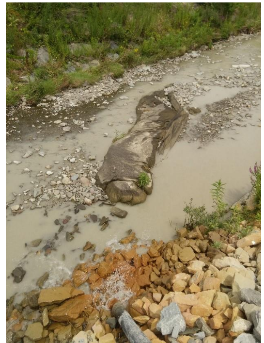
Job site dewatering without use of specified silt-trapping control
