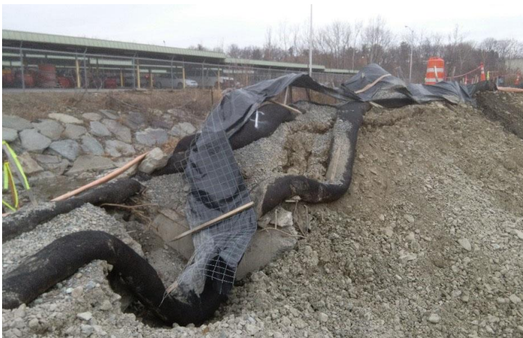
Silt fence and compost filter sock damage adjacent to waterway
