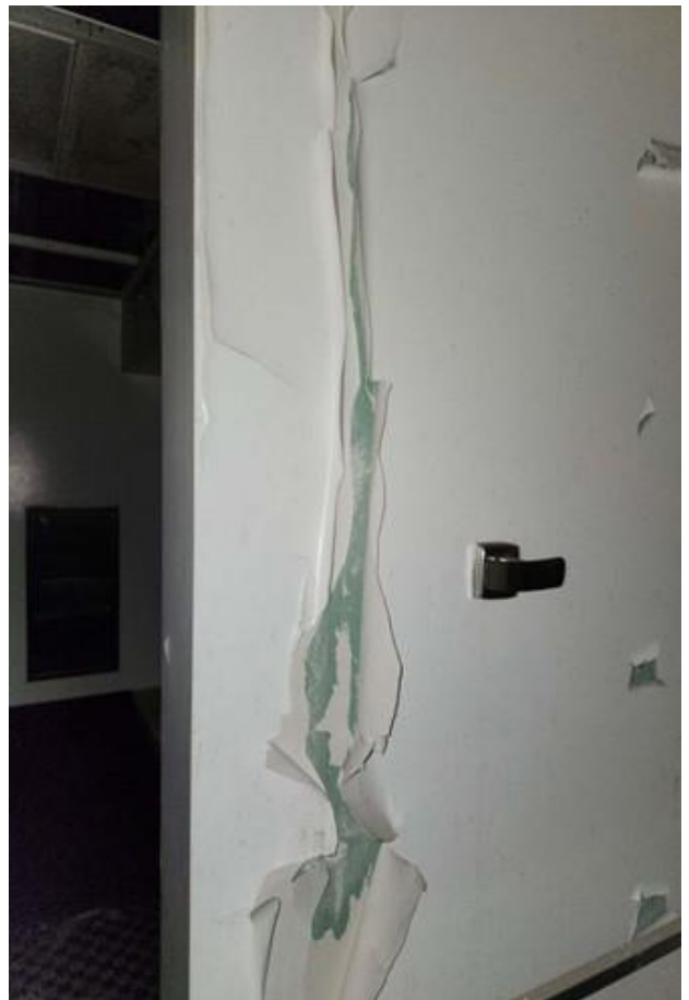
Water-damaged and peeling lead-containing paint.
