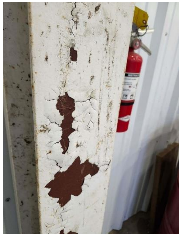
Deteriorating lead-containing paint.
