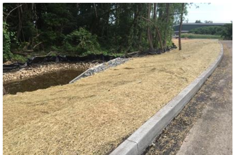
Construction Sequencing: Rolled straw seed blanket installed following final grading of topsoil.
